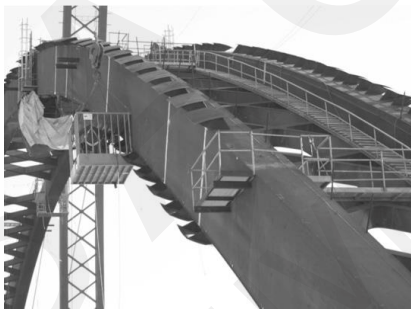
Figure 4. Deflectors on the Alconétar bridge [Corriols A., Morgenthal G. (2012)].
