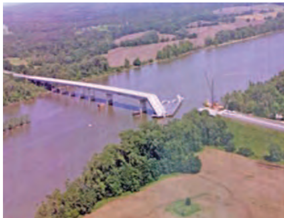
Figure 1.2: Collapse of I-40 highway bridge after being hit by two barges on 26 May 2002 [11].
