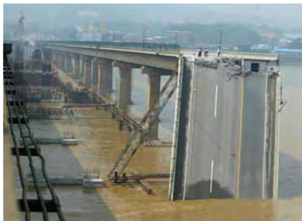
Figure 1.3: Collapse of Jiujiang Bridge after being hit by the cargo vessel on 15 June 2007 [11].
